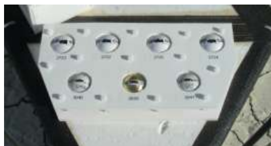
Pongsat may have power on switches.
